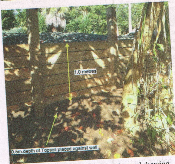
Two views of a wall halfway along the road showing, top, the original 1.5 metre height of the retaining wall and, above, the same stretch after topsoil had been piled up to reduce the height to a metre.
